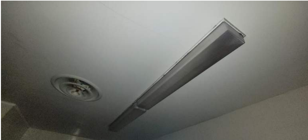
Photo 18-21 Changeroom light fixtures to be replaced
