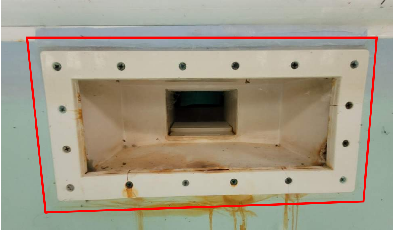
Photo 12 Skimmers to be replaced
