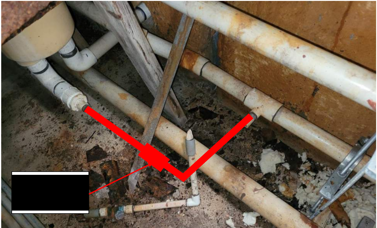
Photo 13 Check valve and piping to be replaced
