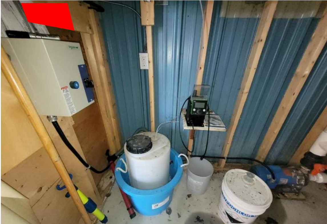
Photo 16 Install exhaust fan to improve chemical storage ventilation and install automated chlorine system
