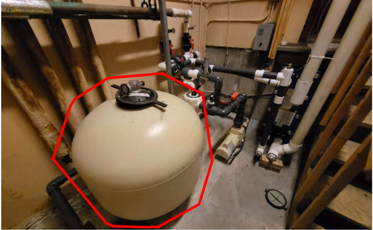
Photo 3 Sand filter to be inspected, existing sand removed and replaced with new and routine maintenance completed
