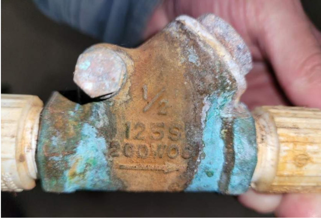
Photo 14 Check valve to be replaced
