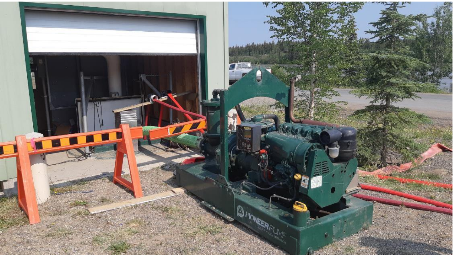
Photo 4. Wastewater lift station adjacent to River Drive and diesel pump as emergency backup, 28-JUN-2022.
